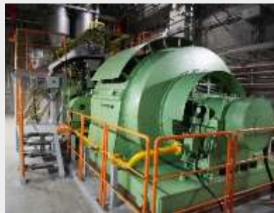
Emergency diesel generators (Two each in Units 1, 2, and 3 since construction)
