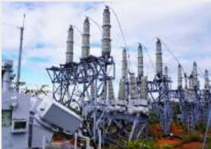
Multiplexed external power supply for Unit 3
