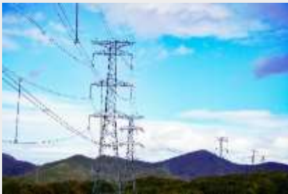
External power source (received from power lines)
