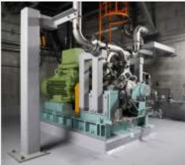
Alternative containment Spray pumps
