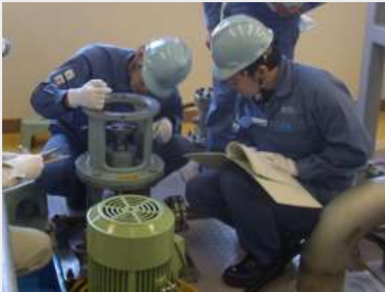
Training of maintenance personnel
