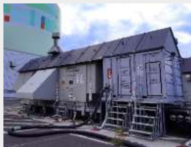
6 units of alternative emergency power supply (permanently installed)
